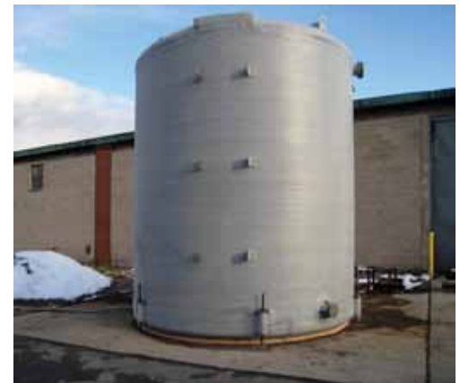
Water treatment plant storage tanks An-Cor Industrial Plastics Vipel® K022 Vipel® F010
